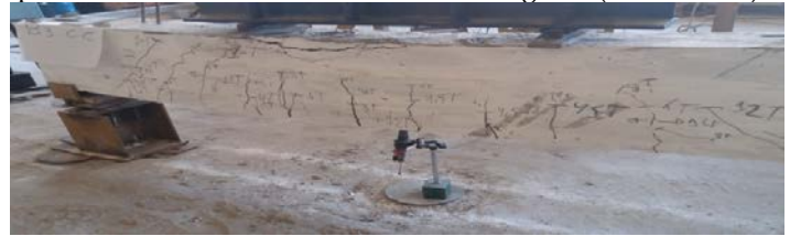
FIGURE25: CRACK DISTRIBUTION FOR RAC BEAM
