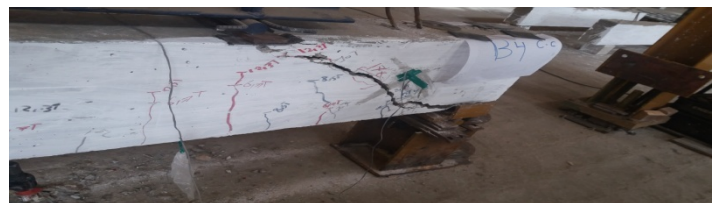
FIGURE29: CRACK DISTRIBUTION FORRAC1 BEAM
