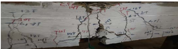
FIGURE33: COMPRESSION FAILURE FOR S.S BEAM
