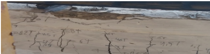
FIGURE32: COMPRESSION FAILURE FOR RAC BEAM
