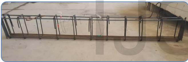
FIGURE 3: BEAM SHEAR FAIURE
